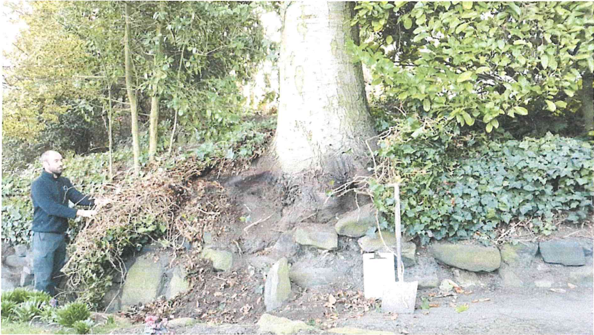
T1 Fir: Showing damage to retaining wall and lack of lateral roots.
