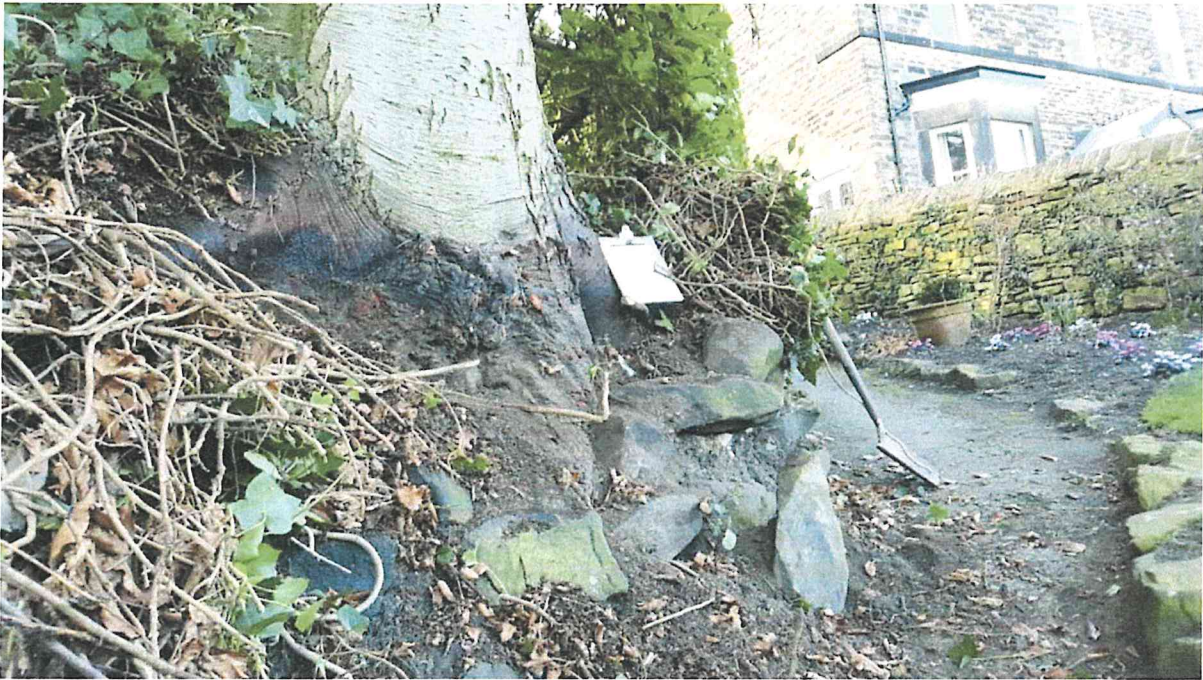
T1 Fir Showing damage to retaining wall and lack of lateral roots.
